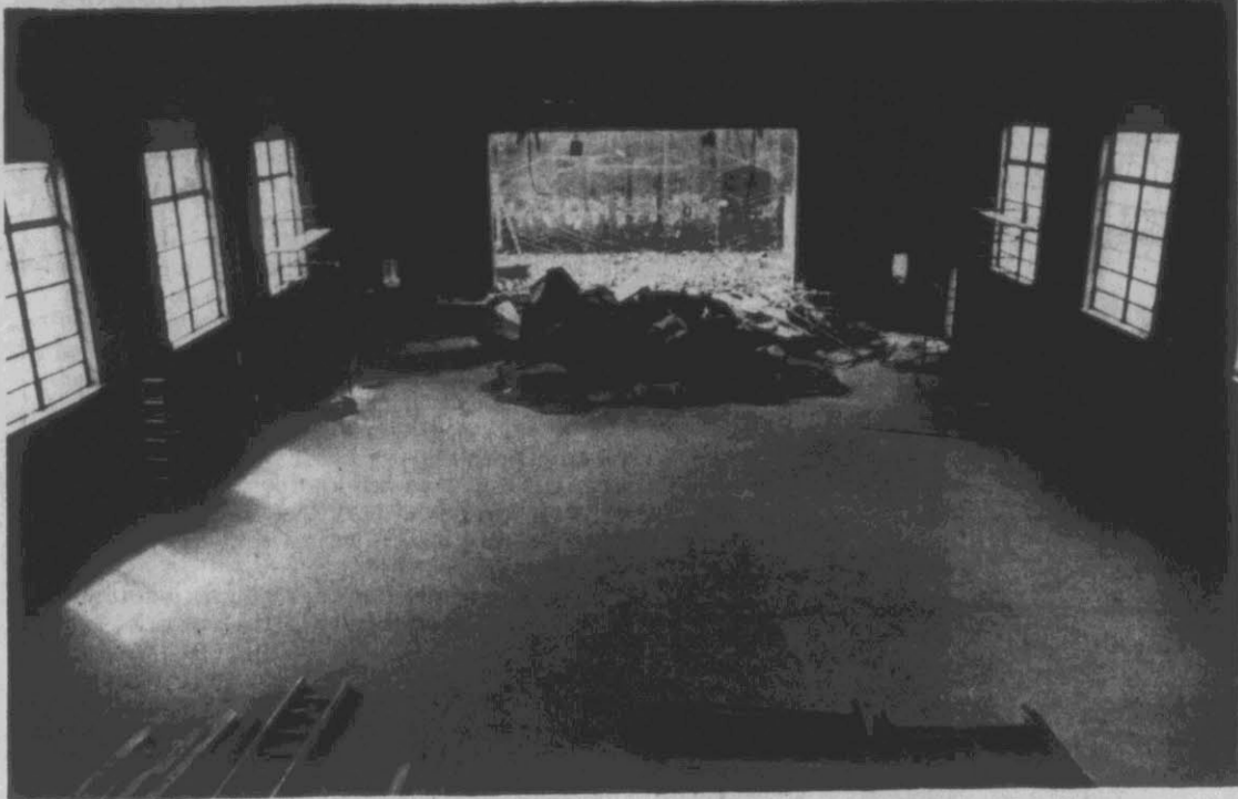
MCGINNIS AUDITORIUM RENOVATION BEGINS — Workers began demolishing McGinnis Auditorium recently in preparation for the construction of a new stage house, which is four times larger than the older one, orchestra pit, dressing rooms, and an elevator. The building was originally constructed in 1951 at a cost of $362,000. The cost of the renovations is said to be approximately
