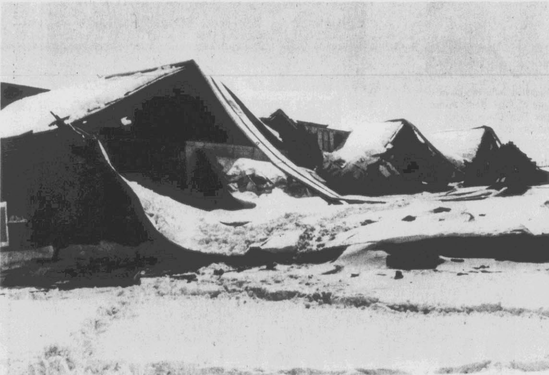
NOT MUCH LEFT. . . Only a small portion at the front of the New Carolina Warehouse at 1700 Dickinson Ave. was left standing after the weight of snow on the roof caused the building to collapse.
