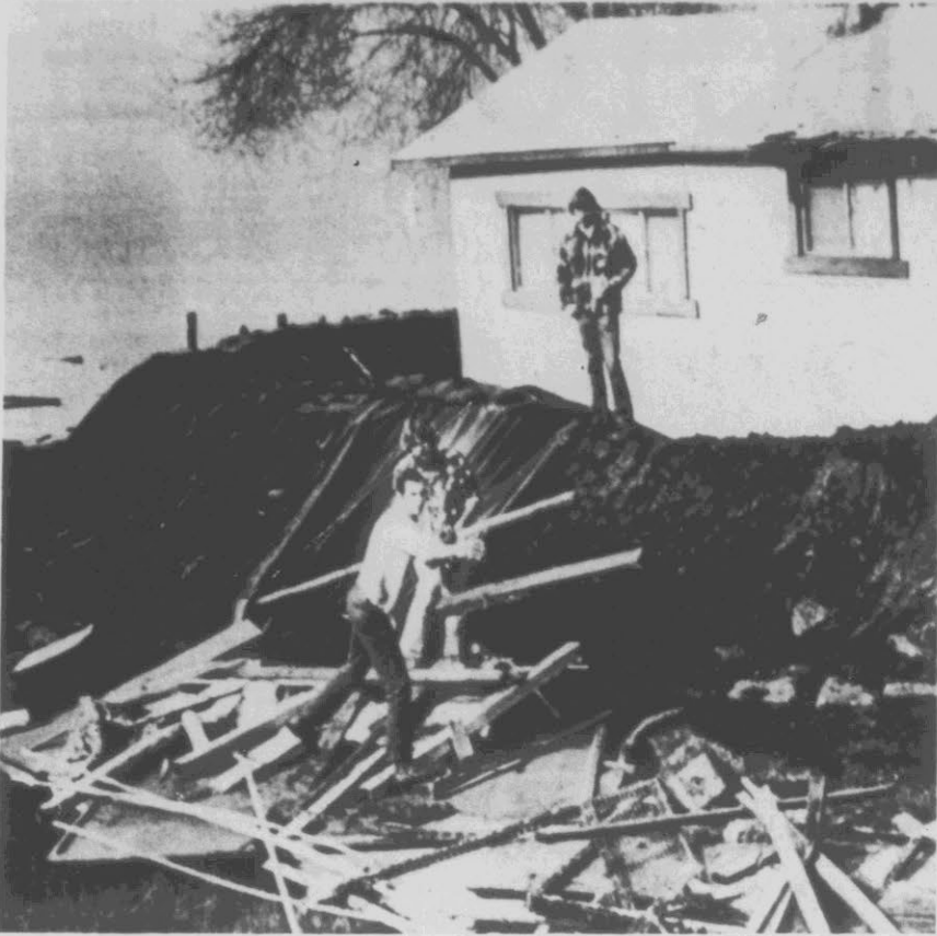
DESPERATE BATTLE — Three men work on makeshift levee around home on rapidly rising Lake Elsinore near community of same name in southern California Sunday afternoon. An Army Corps of Engineers spokesman said the lake was rising at the
