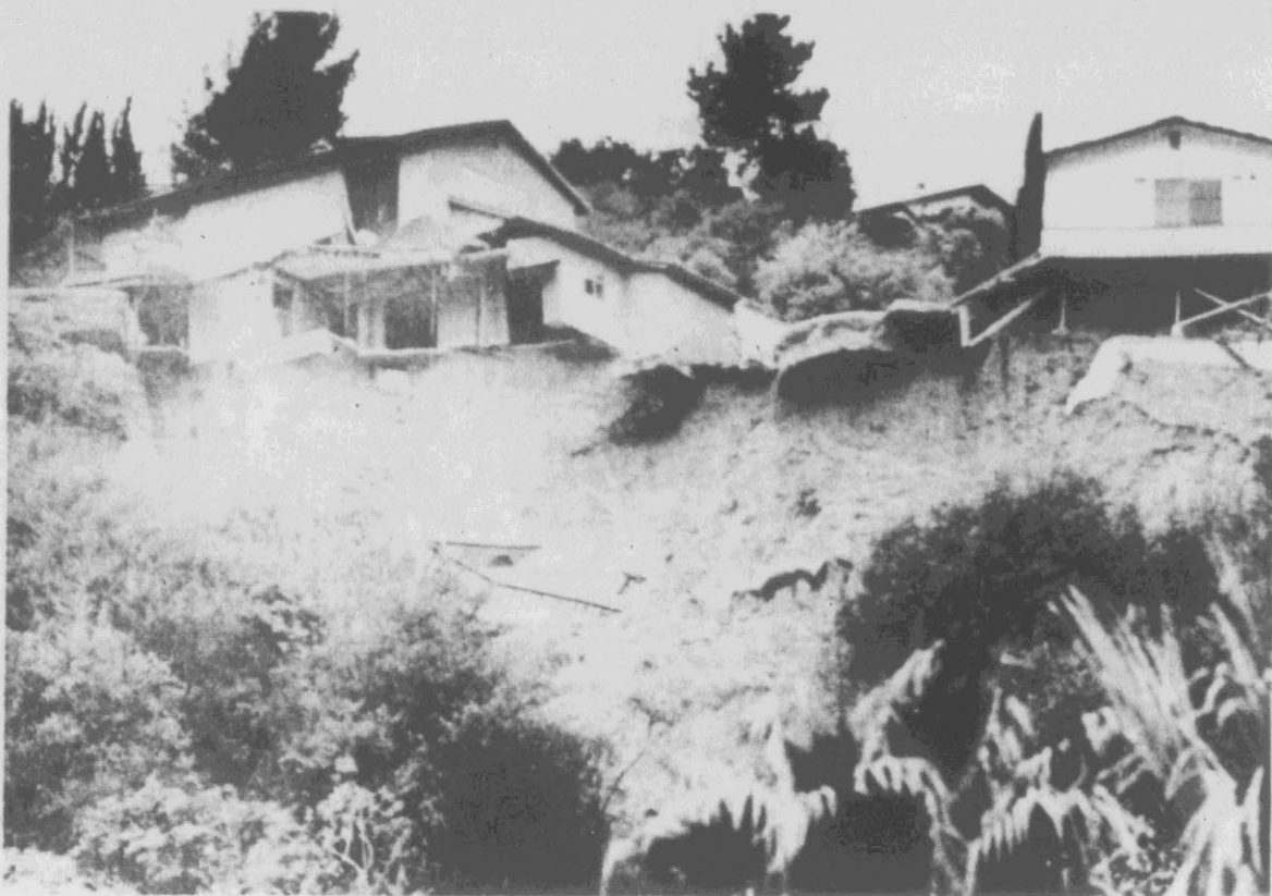
PRECARIOUS PERCH — Rear of house at left hangs precariously over section of washed-away hillside in Stone Canyon section of Los Angeles
