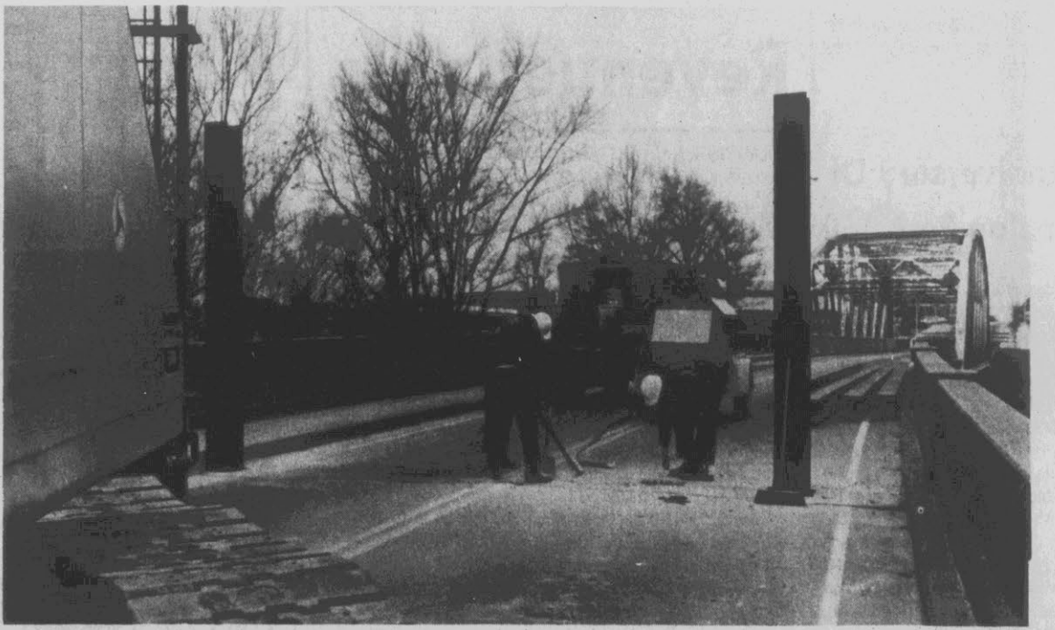
BRIDGE REPAIRS ...North Carolina Department of Transportation Division of Highway's employees are shown working on the Greene Street bridge, north of the span crossing the Tar River. Six pilings
