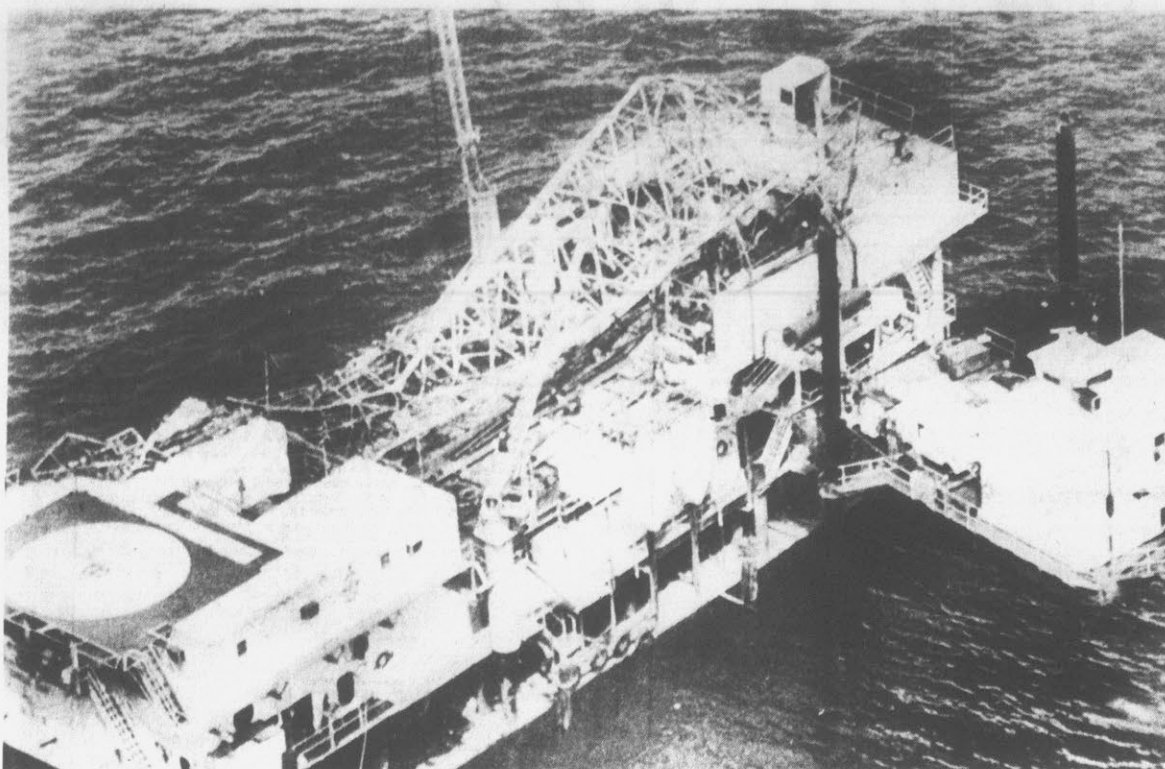
OFFSHORE RIG COLLAPSES — one man was killed and three injured Wednesday when the derrick on this offshore rig collapsed. The accident occurred 25 miles out in the Gulf of Mexico in Vermillion Block 32, just south of the oil community of Intracoastal
