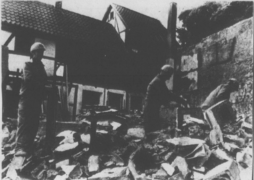
TREASURE HUNT —Polish experts look for usable brickwork while restoring a half-timbered house in Bonn, West Germany. Polish restorers became world leaders in the field by rebuilding beautiful old cities in their country and abroad.
