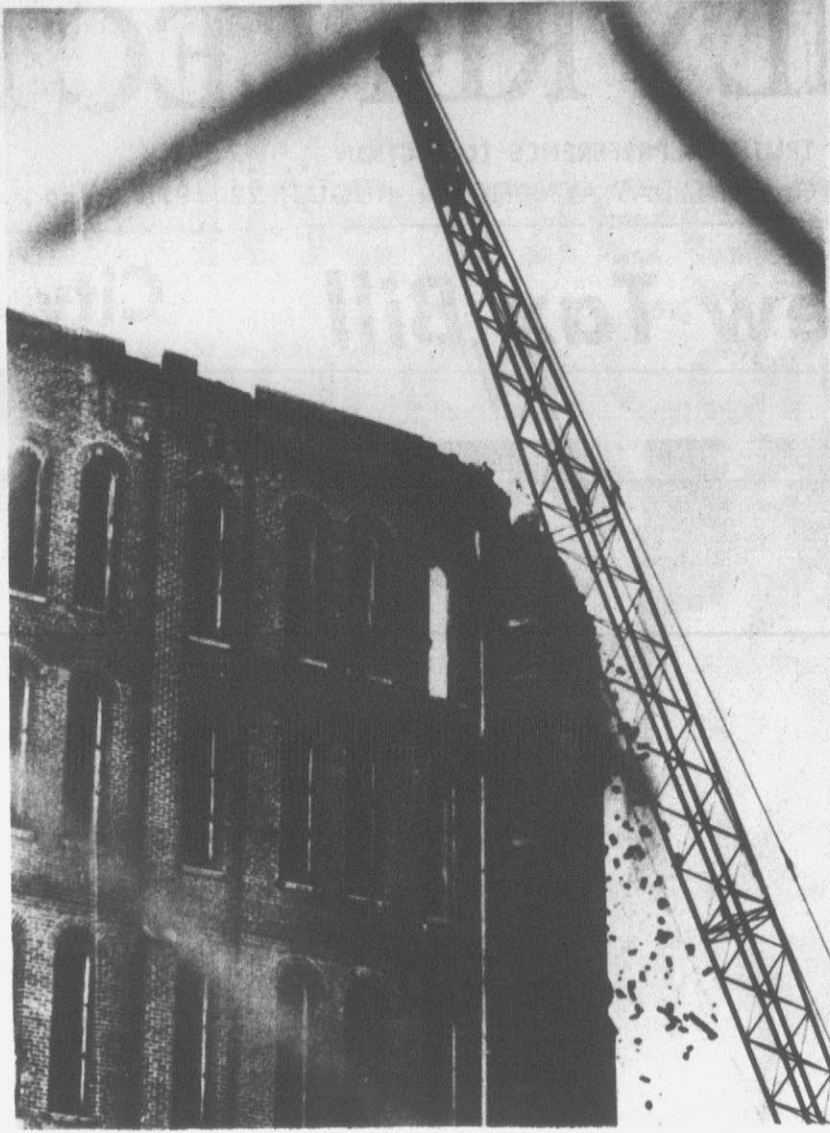
DEMOLITION BEGINS — Wrecking crews began the first stage of demolition on the oldest buildings at Central Prison in Raleigh Monday. The old buildings will be replaced with new
