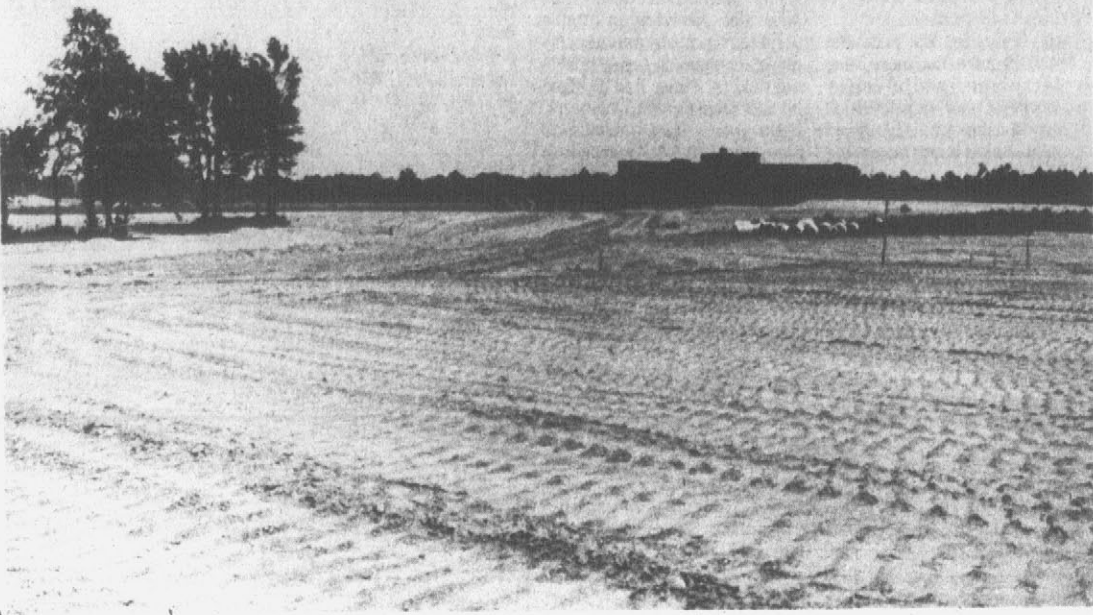
CLEARING LAND — Construction workers prepare land for the new East Carolina University medical school complex. Construction is expected to begin after the first of the year. The new complex will have about 450,000 square feet and will cost approx-
