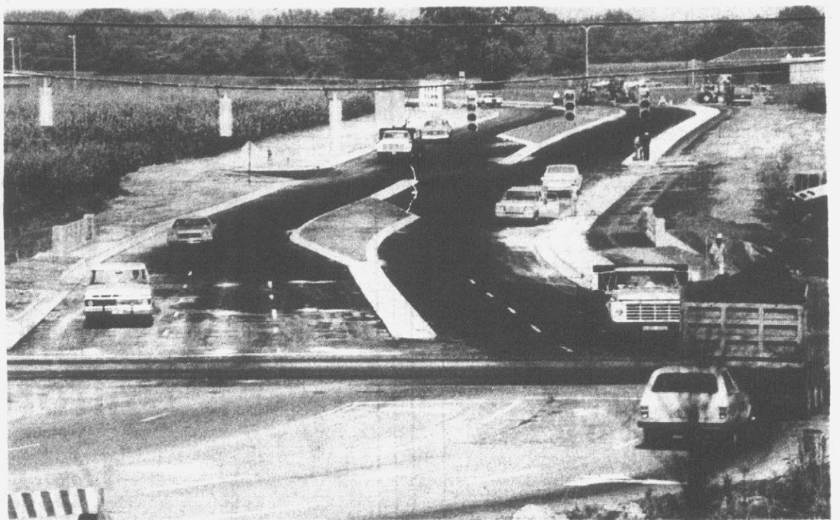
NOW OPEN . . . The new segment of Arlington Boulevard from Evans Street to Hooker Road was opened to traffic Monday. This photo shows a view
