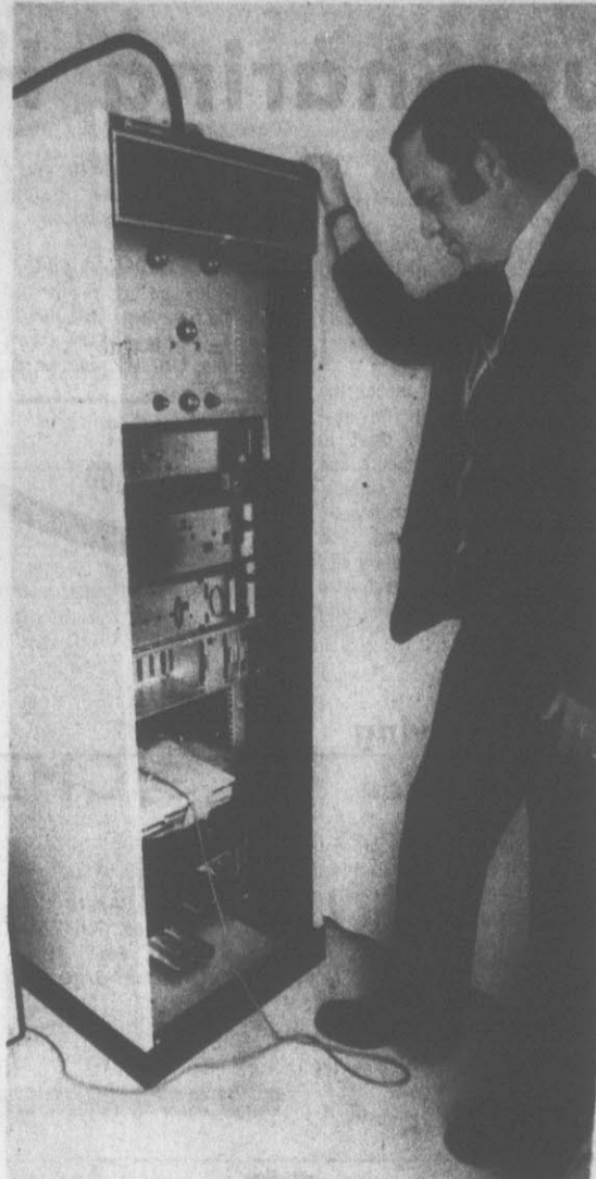
TRANSMITTER INSTALLED — Greenville Utilities Assistant Director Malcolm Green looks over the new transmitter that will be used to transmit signals controlling the load management switches that have been installed in homes in the Pitt County area. The signals will switch receivers that control hot water heaters and air conditioners during peak demand hours when Greenville Utilities is on a demand charge from Virginia Electric and Power Company. (Reflector Photo by Tommy Forest)
