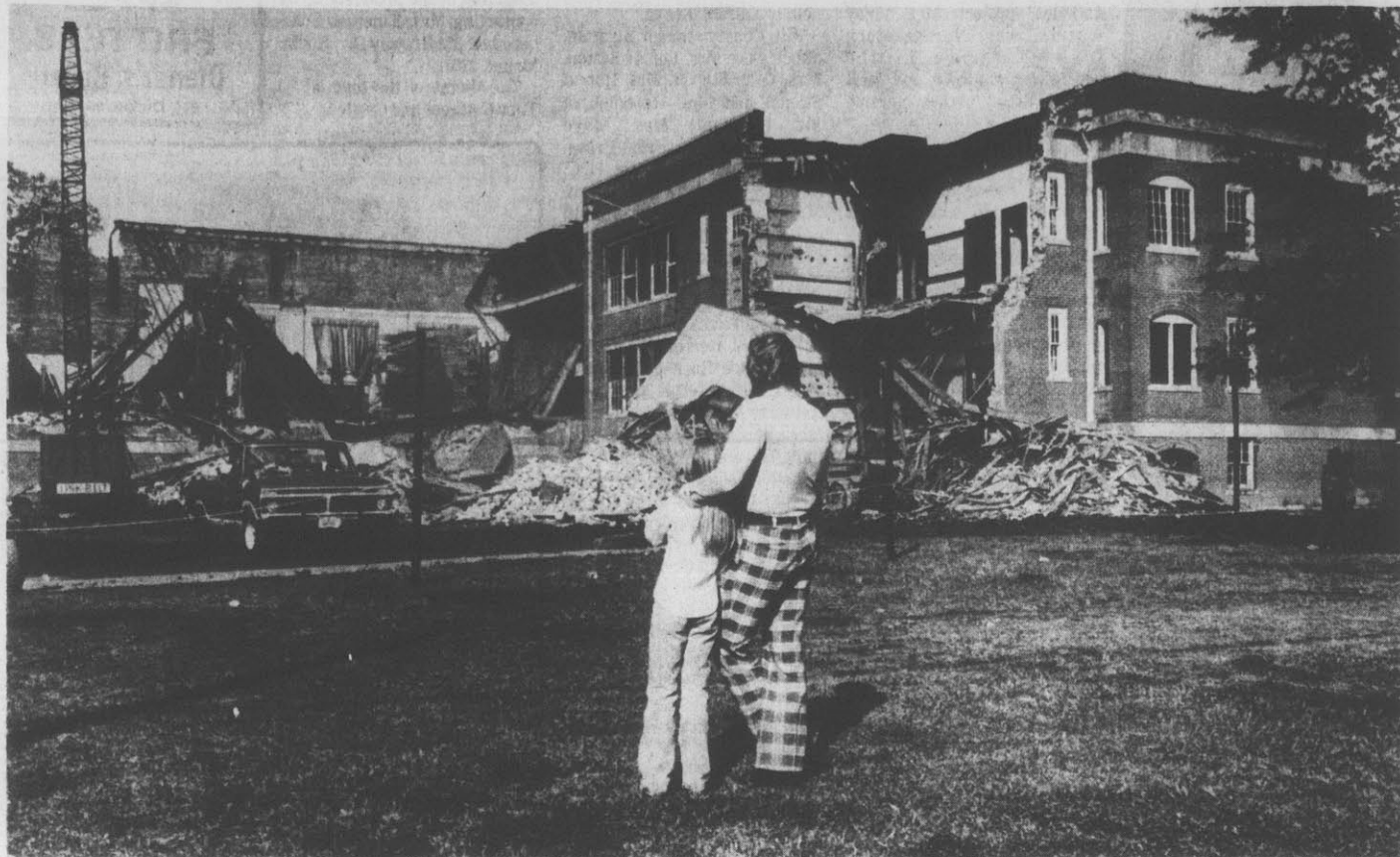
"THERE GOES DADDY'S SCHOOL" — 1947 Farmville High School grad Bill Gregory tells his daughter as the two watch demolition of the 57-year-old building. (Reflector Photo by Carol Tyer)
