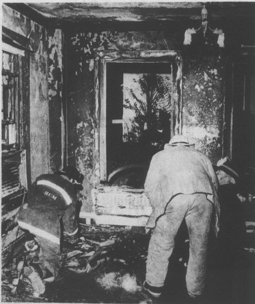
BURNED ROOM — Greenville firemen look through debris in an attempt to determine the cause of a fire which heavily damaged the living room of a house at 108 South Harding St. about 4:26 a.m. today. Heavy smoke damage resulted to the two-story wood-frame dwelling along with
