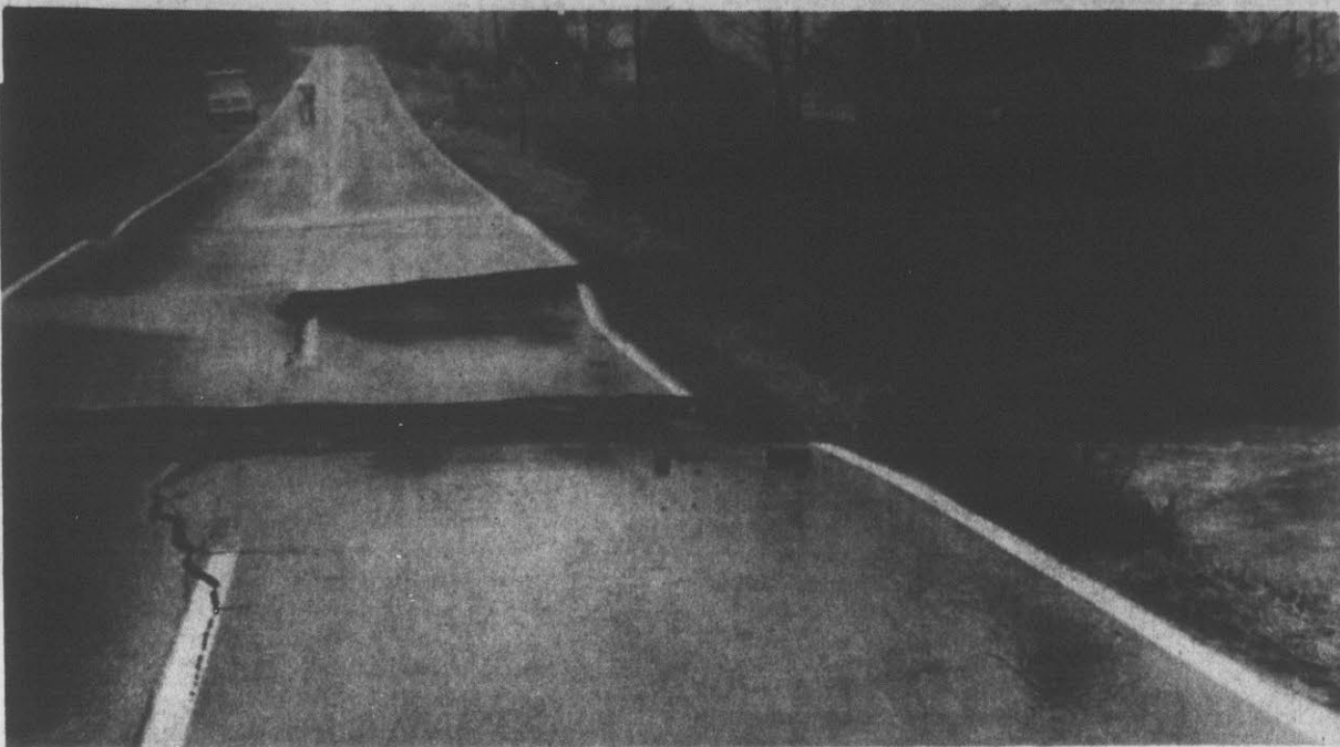
BOTTOM FELL OUT — A creek swollen by heavy rains washed away this section of U. S. 421 about 12 miles west of North Wilkesboro, N. C., Sunday as
