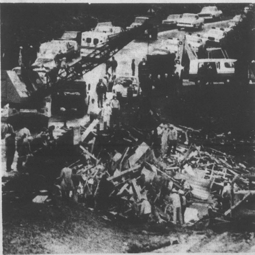
BRIDGE BLOCKED — Debris is cleared from under a bridge at Toccoa, Ga. Sunday after an earthen dam burst and water flooded the Toccoa Falls Bible College campus and an area of
