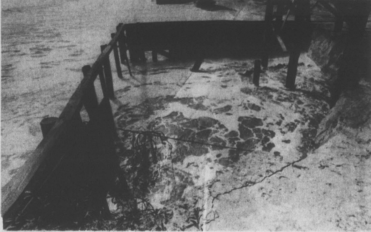
EROSION MENACES BEACH COTTAGE — Rough seas and an extreme high tide erode huge chunks of berm from areas of Wrightsville Beach. Here the water has washed out the bulkhead protecting a cottage. (AP Laserphoto)
