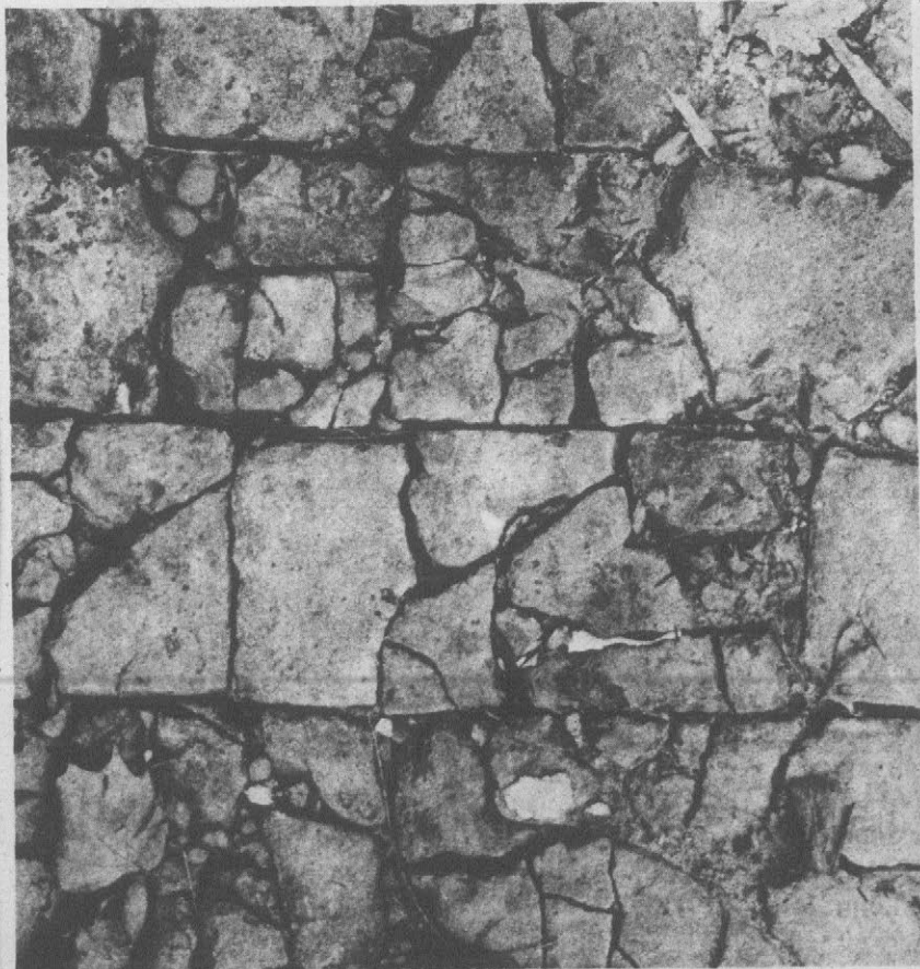
...crumbled bricks in an old pathway...
