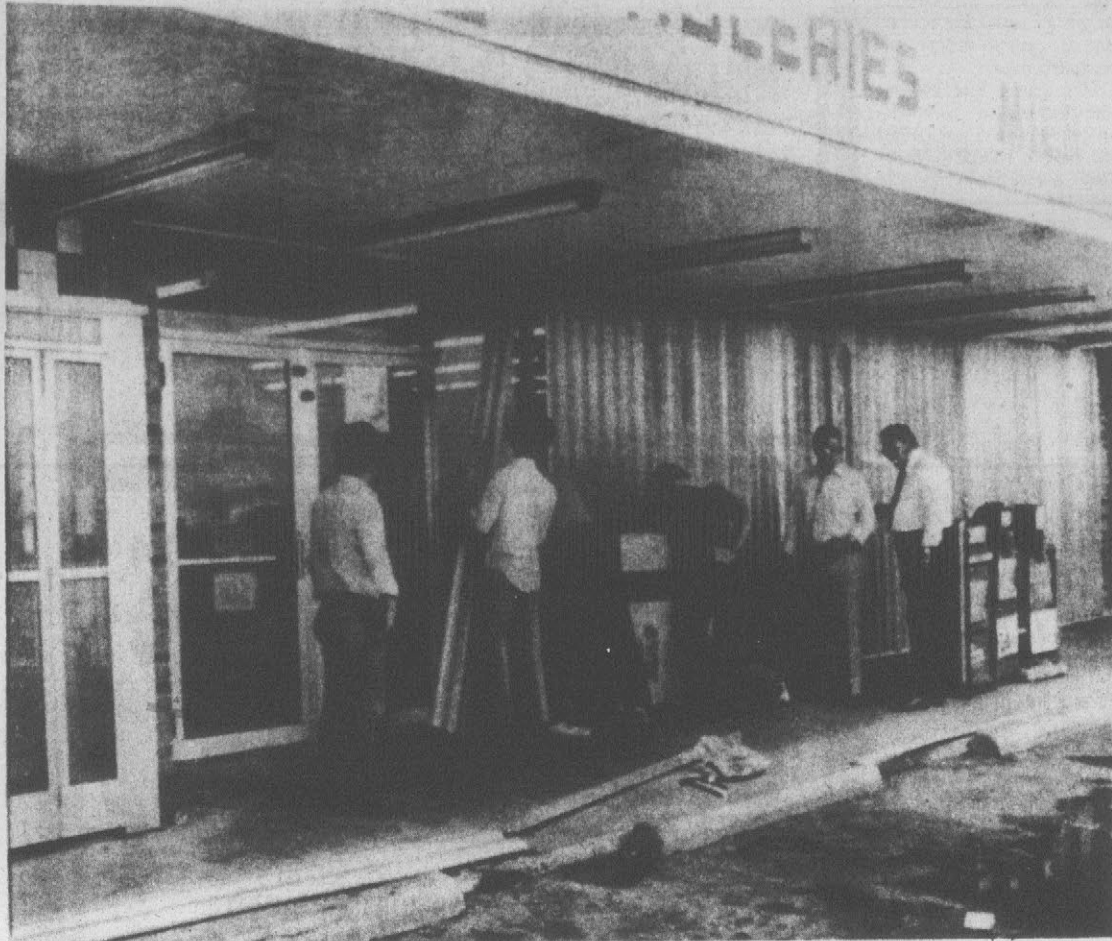
STEELING UP — Workmen in Galveston use corrugated steel to cover the glass front of a store as
