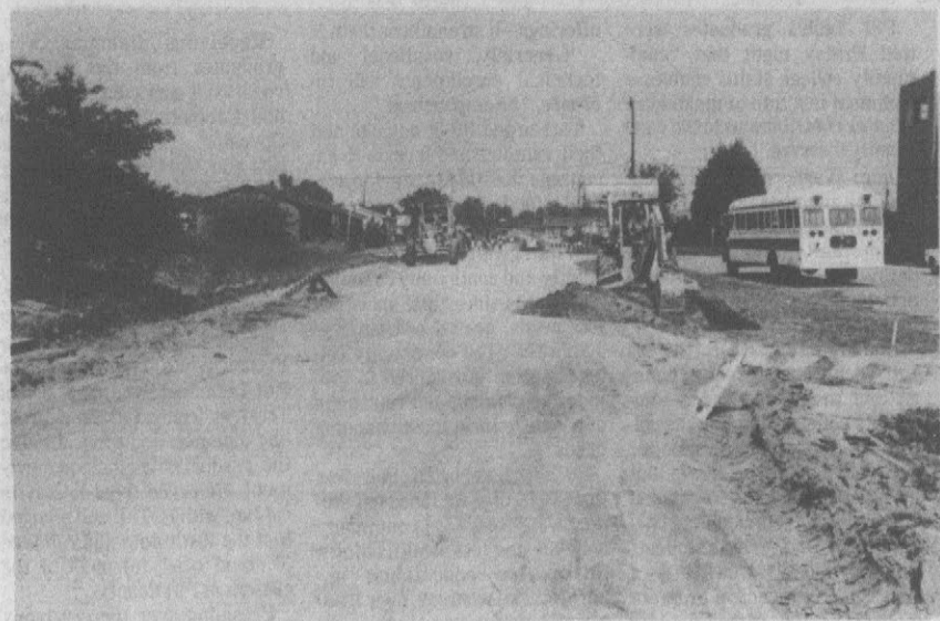
WORK PROGRESSES...City workmen progress on the installation of curb and gutters on Halifax Street, one of several in the West Greenville area
