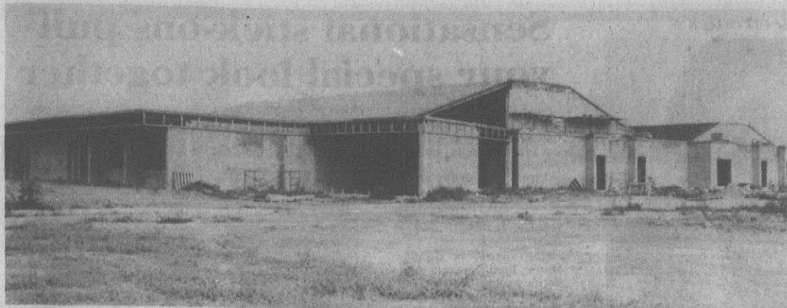
NEW MIDDLE SCHOOL PROGRESSING —work on the new middle school is progressing, according to city school officials. If all
