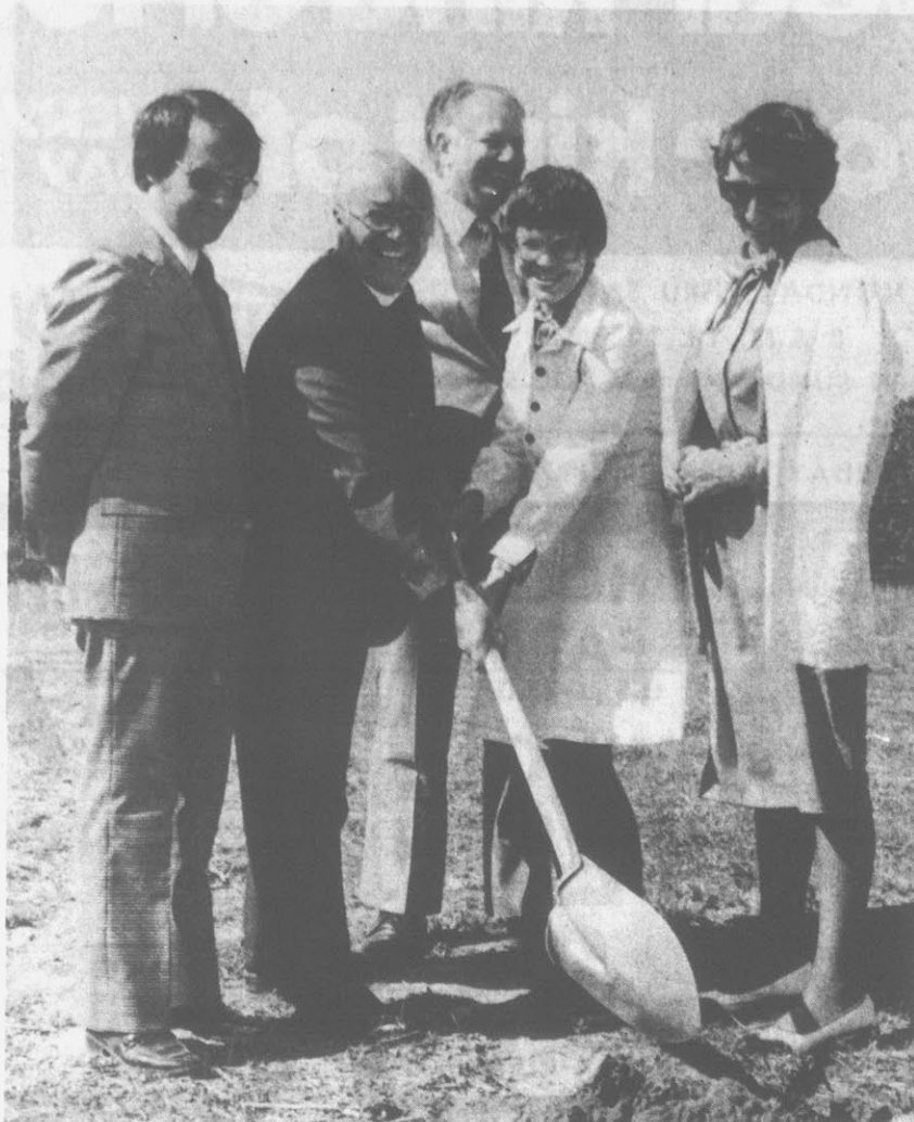
GROUNDBREAKING — for the joint Library-Recreation Building, to be located at Jaycee Park in Greenville, took place at 10 a.m. today. Participating are (left to right), Boyd Lee, director of Greenville Recreation and Parks Dept.,
