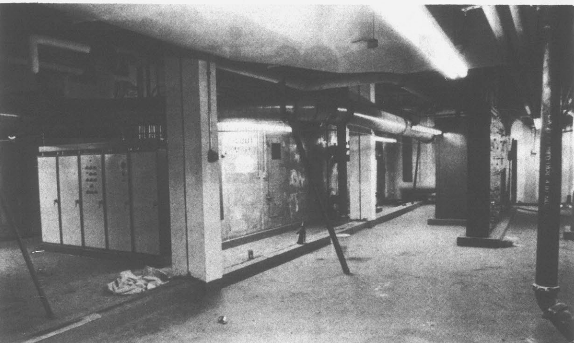
AIR HANDLING UNITS —Large units in the upper portion of the new Pitt Memorial Hospital move air throughout the building. These units purify air and are controlled by the central computer, as to the amount of humidity and temperature. The complete system can be monitored, even the condition of the filter. (Reflector Photo by Tommy Forrest)
