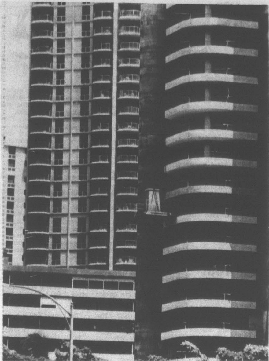
HIGHRISE OUTHOUSE — Construction is construction, and the law is the law. So this outhouse was installed in the middle of a highrise building
