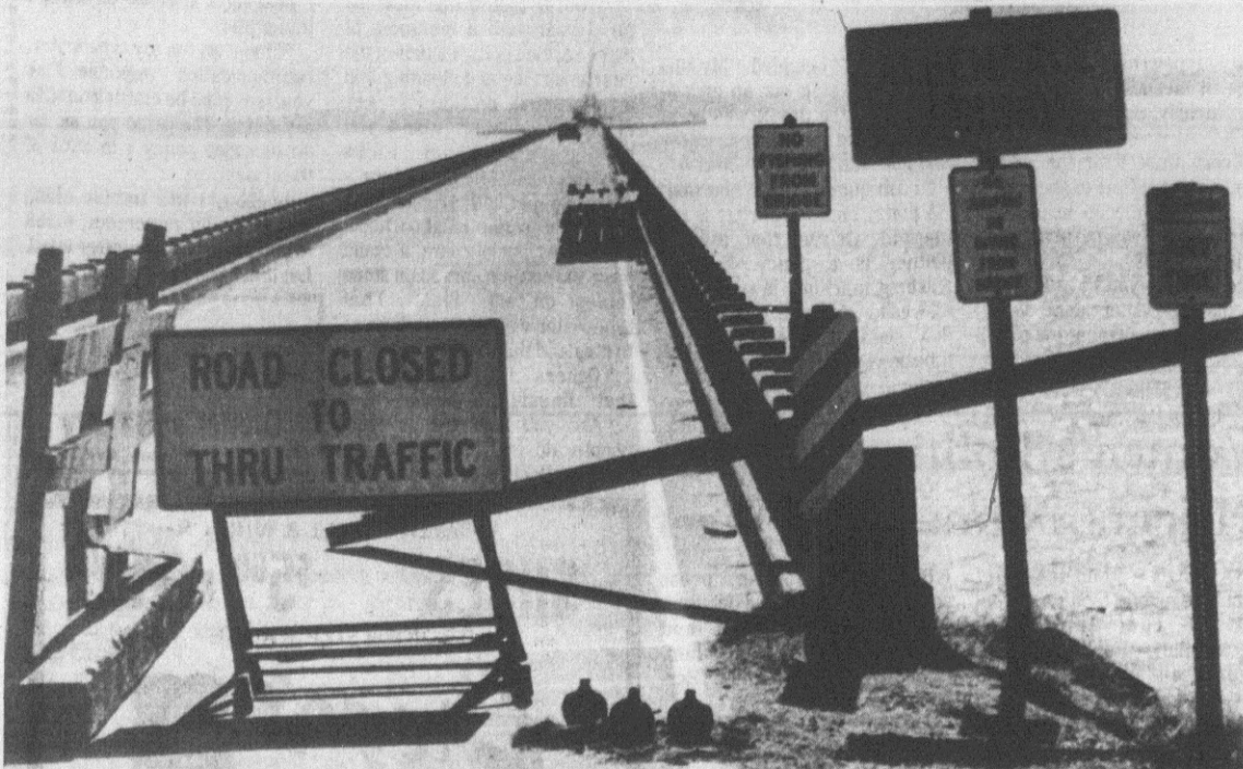
BRIDGE CLOSED BY ICE — The Albemarle Sound Bridge, which connects Chowan and Washington counties on Highway 37, has been closed since ice severed 46 of the piles that support the span. The
