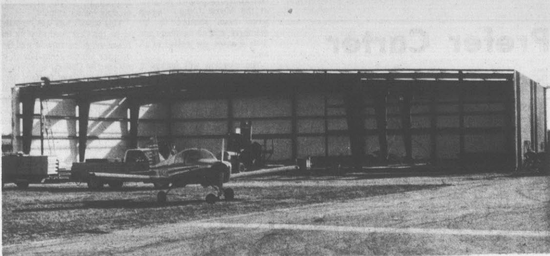
NEW HANGAR ... A private plane sits in front of a new hangar under construction at the Pitt-Greenville airfield.
