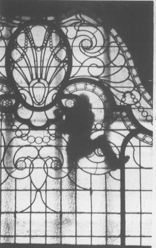
A REAL PANE — Silhouetted against the object of his labors, a worker slowly removes a pane of stained glass from a large lobby window in Cincinnati's historic Albee Theatre. The theatre, which was opened in 1927, is being torn down to make way for a new office building complex. The stained and leaded glass, which has to be removed one pane at a time, has been purchased by a glass dealer who plans to resell the display. Workers estimate it will take two to three days to bring the glass down. (AP Wirephoto)
