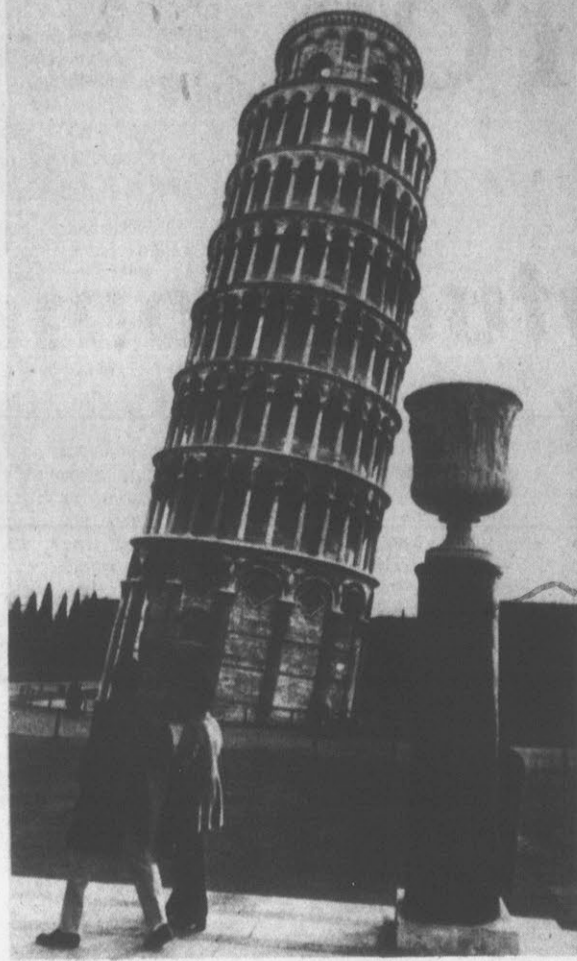
LEANING SLOWER, BUT STILL LEANING — A verticle column with a vase contrast with the Leaning Tower of Pisa in this recent Photograph. Experts in Italy say the famous tower's rate of leaning was slower for the third consecutive year, just over nine-hundredths of an inch, or about half its traditional tip per year in recent decades. (AP Wirephoto)
