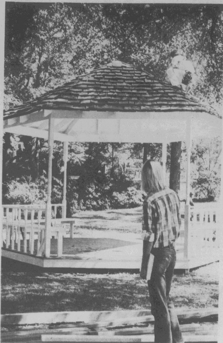
GAZEBO—An East Carolina University student pauses to look as Bill Dill, an ECU graduate from New Bern, clambers atop the gazebo he has designed and built in a special beauty spot on campus. The structure, gift of the Class of '74, will be finished as soon as Dill adds a few more shingles and last minute touches. (ECU News Bureau Photo by Marianne Baines.)
