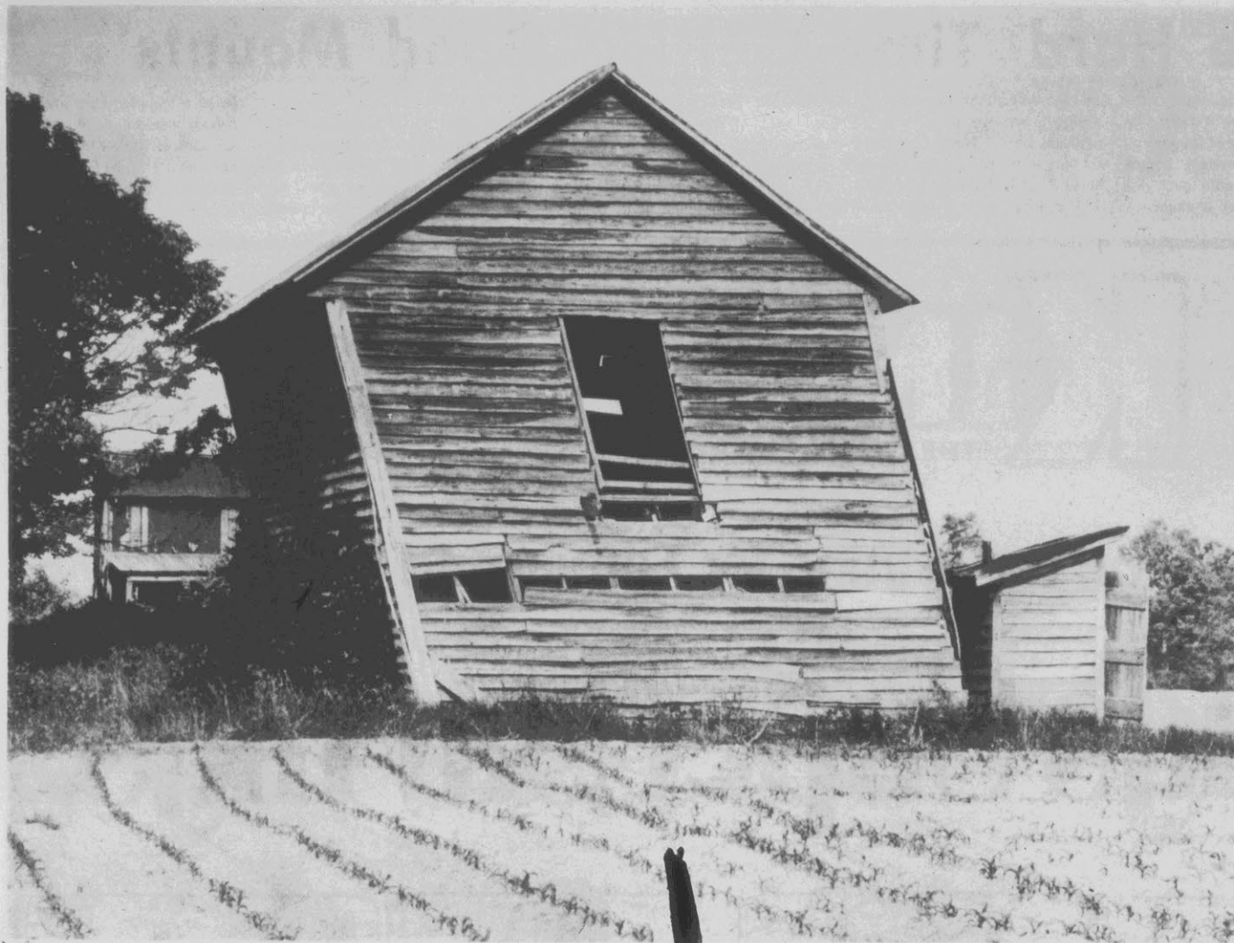
LEANING—This old barn, blown by the wind for years, has finally given away and begun leaning. Its boards are bent with time and a few are missing, here and
