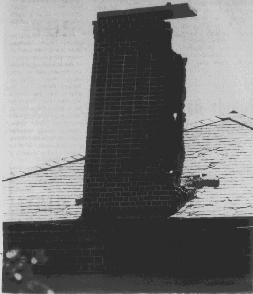
CHIMNEY DAMAGED . . . Workmen began today tearing down a chimney of Sheppard Memorial Library which was severely damaged by lightning about 7:30 p.m. Friday. Structural damage to the north end of the building called for
