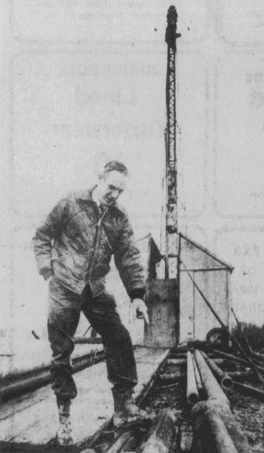
DRILL YOUR OWN WELL — John Cochrane, president of the American Exploration Co., a gas-drilling firm that develops and manages self-help projects for industry, stands in front of a well his company is drilling for Ohio Elevator near Somerset, Ohio. Like other firms, Otis must work out an agreement with the utilities for the taking in of gas at the utility's station nearest the wells and the displacement of it at a specified plant. In this case the well is far removed from the plant. (AP Wirephoto)
