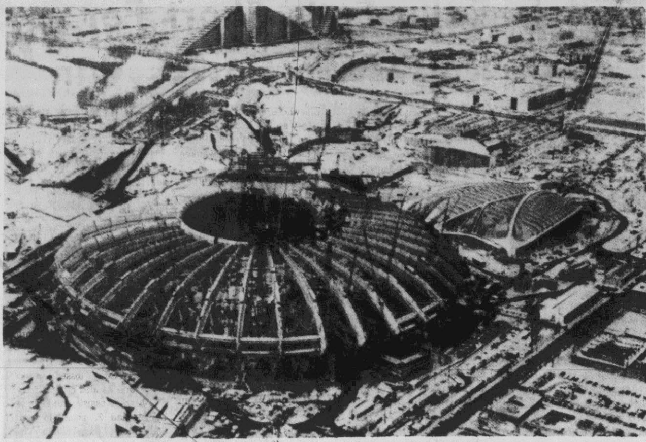
WORK CONTINUES — Barring any further construction halts, the 1976 Summer Olympic Games will be held in Montreal as scheduled, Quebec Minister of Municipal Affairs announced Wednesday. But, what was to be one of the most spectacular stadium in the
