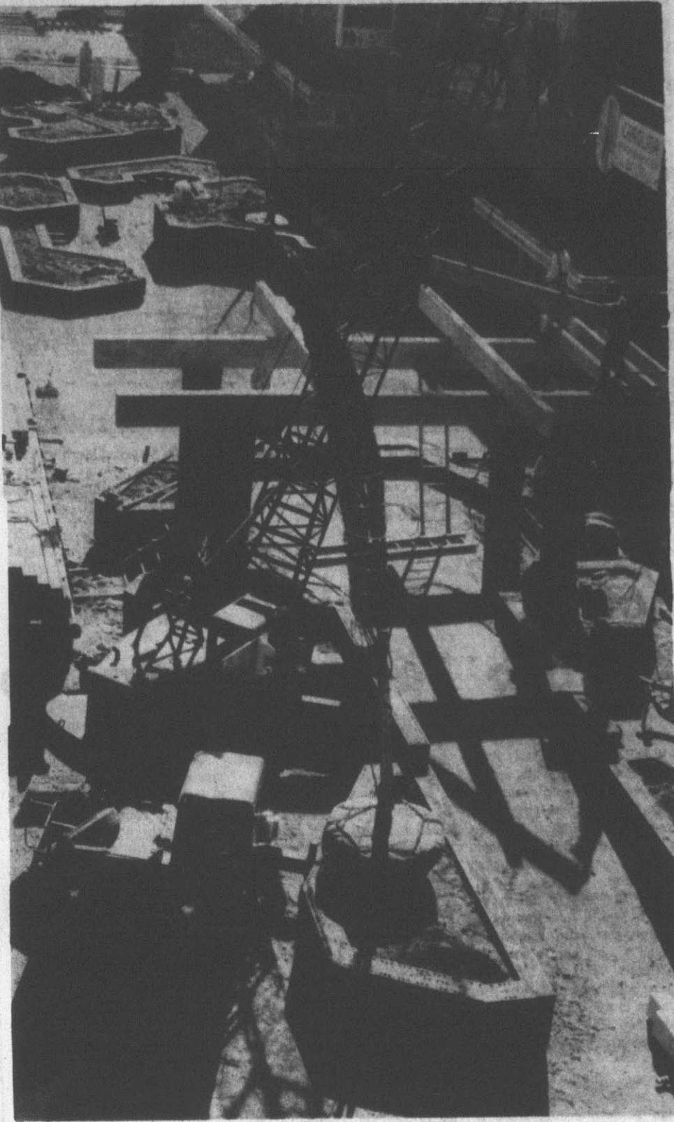
Weighty Lift Is Involved HEAVY WORK... involving the bulky overhead slabs. (Reflector Photo by Stuart Savage) requires the use of a crane to lift the
