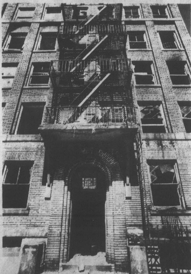
Windows gape, once sturdy building begins to crumble.
