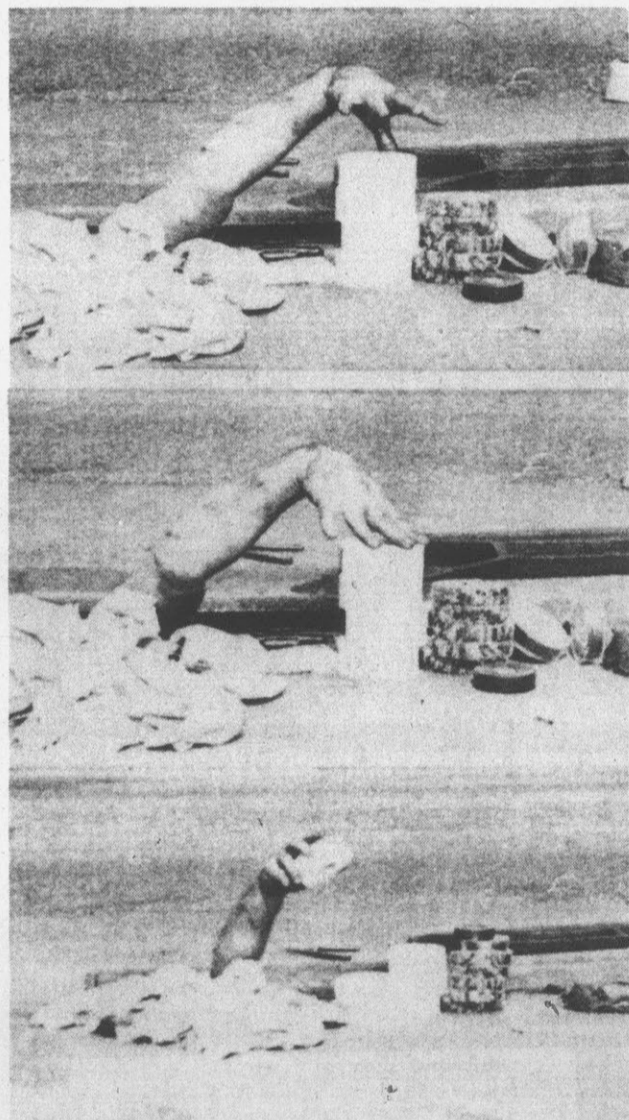
THE HAND FROM DOWN UNDER —The hand of an electrical company worker seems to be reaching out from the depths of the earth, like a monster reaching for a snack. Actually he is reaching for a roll of tape used to repair underground conduits making them moisture proof. (AP Wirephoto)
