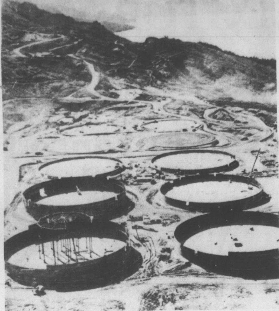
STORAGE FOR OIL —Crude oil storage tanks take shape at the Valdez (Alaska) terminal site for the trans-Alaska pipeline. Eighteen of the half-million barrel capacity tanks will be built to handle the pipeline initial 1.2 million barrels per day. Each tank will hold an internal steel structure being erected in front left tank, to support a cone-shaped roof required for heavy winter accumulations of snow. (AP Wirephoto)
