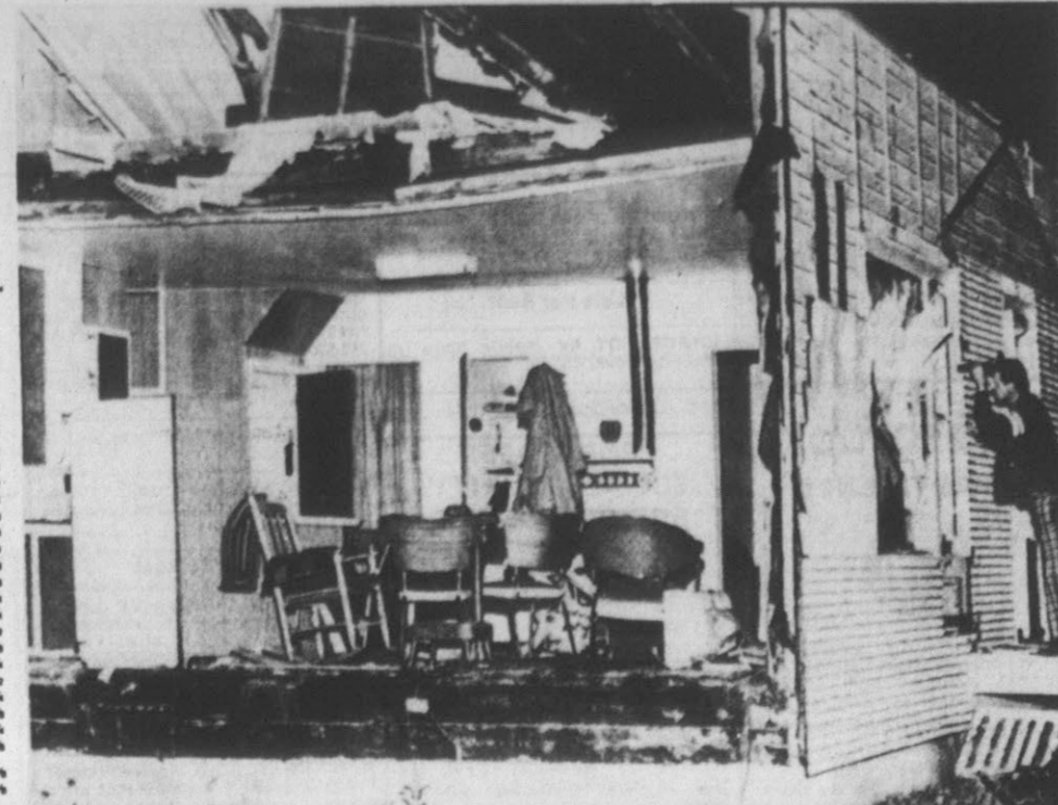
WALL-LESS —A man peers through the door of a house in St. Bonaventure, Que., fifty miles east of Montreal early Friday, unaware that the wall has been sheared away by a tornado, revealing kitchen furniture. The storm claimed the lives of three people. (CP Wirephoto)
