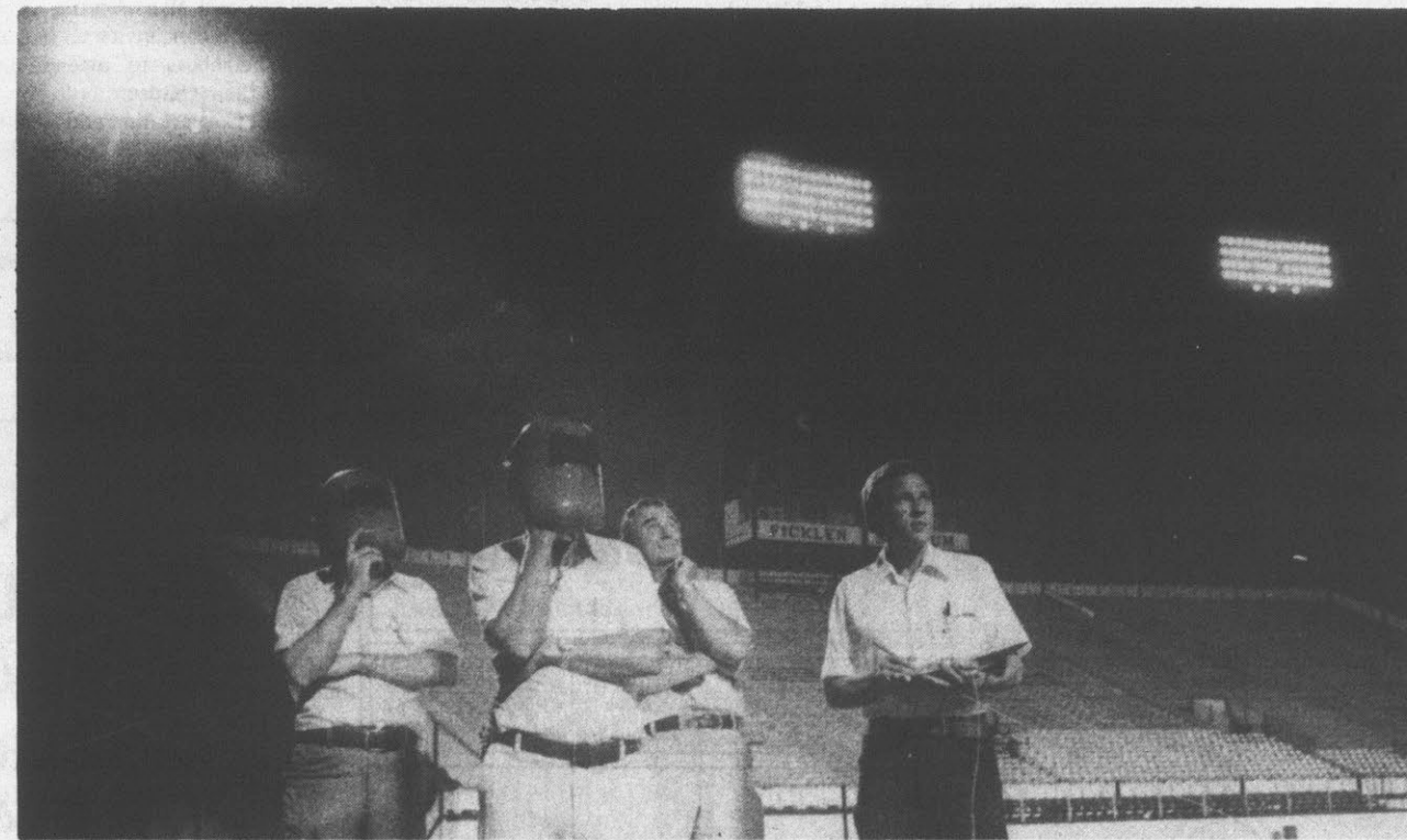
Turning Night Into Day UNDER THE LIGHTS—The new lighting system at Ficklen Stadium was recently installed. To complete the installation are workers above, left to right, John Campbell contractor, Linwood Wall, Newton Simmons, of General Electric which manufactured the lamps; and Dave Wollager, of L.E. Wooten Engineers. Campbell and Wall use welders' masks to protect their eyes while focusing each lamp on the football field. There are 312 lamps, running on 480 volts. The multivapor lamps are on the top of 160 ft steel towers. Each tower weighs, with lights, approximately 35,000 lbs. (Reflector Photo by Tommy Forrest)
