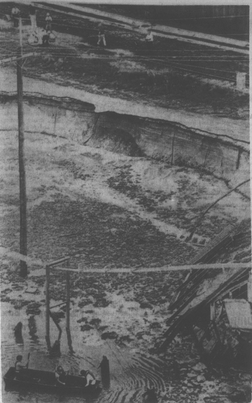
CHECK EXTENT OF LEVEE COLLAPSE—Member of the U.S. Corps of Engineers check damage to a 150-foot section of the levee that collapsed along the Mississippi River at New Orleans Monday. A partially collapsed shed is at right while levee sand continues to drop off into the river, posing a threat to huge grain elevator behind the levee. (AP Wirephoto)
