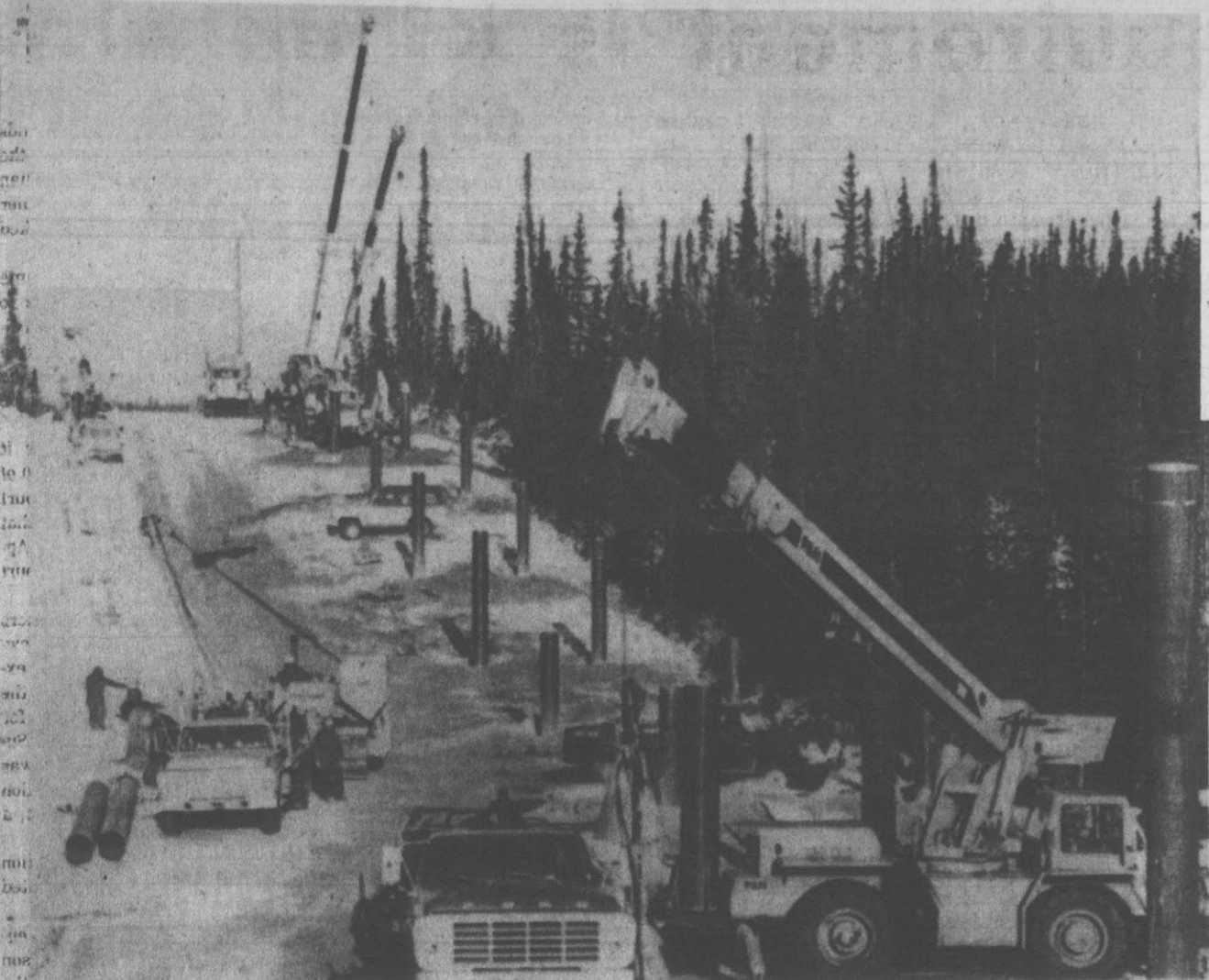
ALASKA PIPELINE CONSTRUCTION—Just north of the Yukon River, crews install pairs of supports for a section of the trans-Alaska pipeline which will be installed above ground. A cross beam will later be placed between the 18-inch diameter supports. Some 70,000 supports will be needed on construction of the oil pipeline. (AP Wirephoto)
