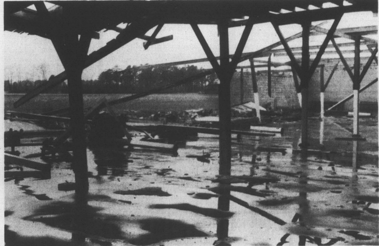
HIGH WINDS... ripped out sections of roof and about 60-feet of cement block wall at Raynor-Forbes-Clark Warehouse on Dickinson Avenue about 4 p.m. yesterday. Damage to the building was estimated at $10,000 to $12,000. (Reflector Photos by Stuart Savage)
