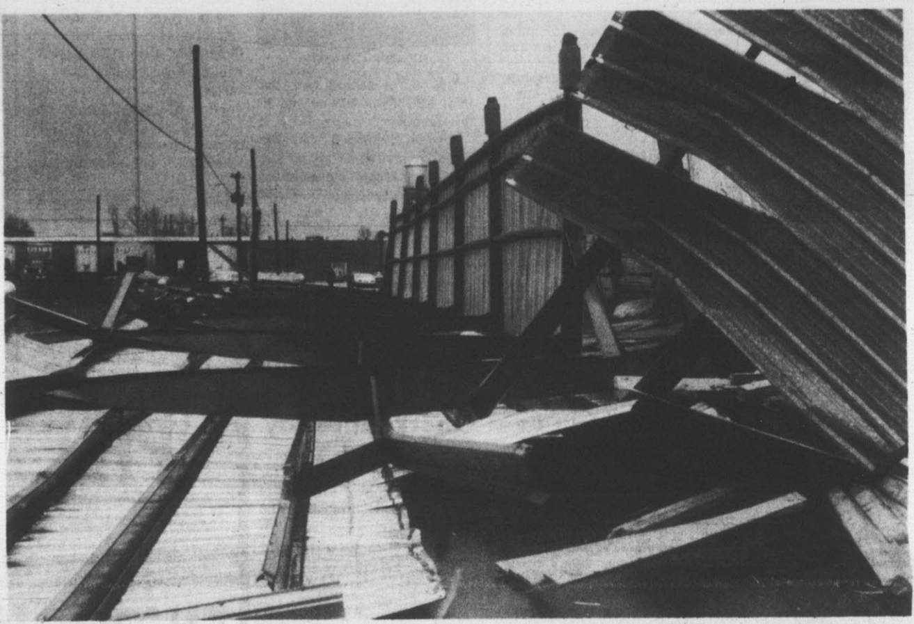
BLOWN OVER... A block-long metal storage shed at Home Builders Supply Co. covers Wilson Street between Chestnut Street and Myrtle Avenue after high winds flipped the structure over. Company officials estimated damage at $30,000 to $35,000.
