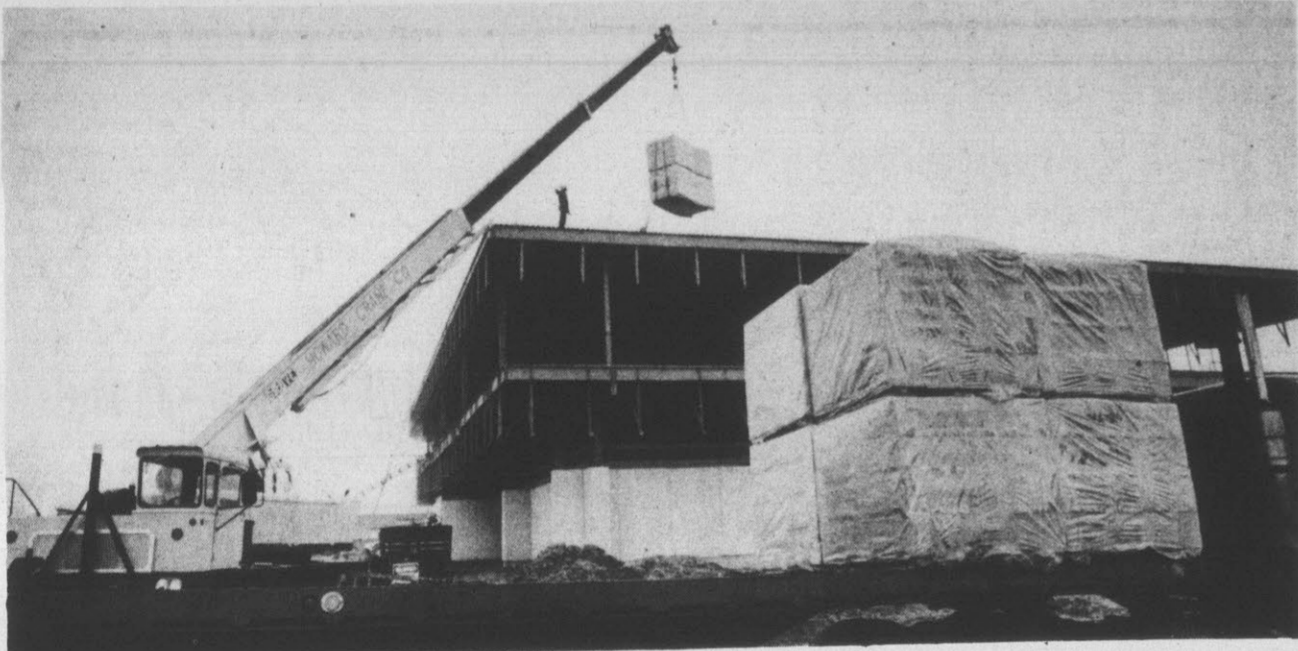
THE BIG LIFT —A crane in the morning fog lifts a 20,000 pound cargo of insulation for the new North Carolina National Bank on Second and Washington Streets. Workers on top of the building position the load in its proper place for installation. (Reflector Photo by Tommy Forrest)
