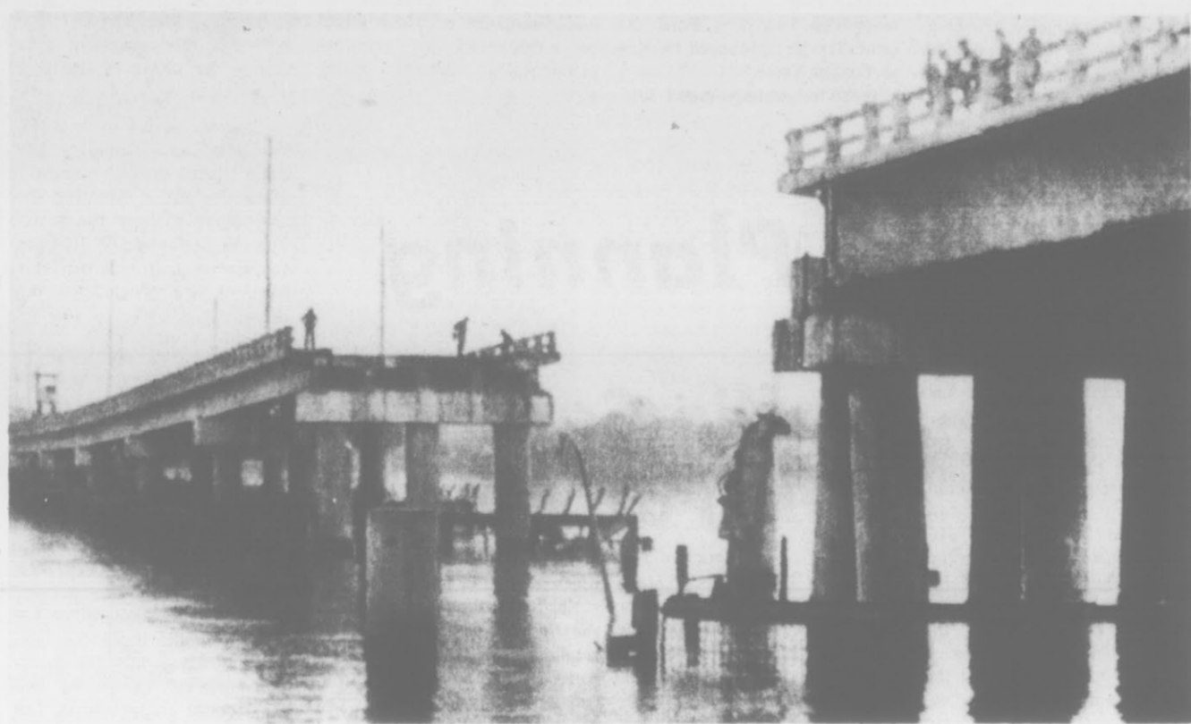
BRIDGE SPAN DEMOLISHED NEAR SAIGON—South Vietnamese government soldiers look down at the wreckage of two spans of the Hoa An bridge near Bien Hoa, some 12 miles north of Saigon. The military command says Viet Cong frogmen using a raft loaded with explosives were responsible. About a dozen bridges have been blown up in the past week and authorities say the Viet Cong are trying to disrupt the economy by isolating cities, towns and villages. (AP Wirephoto)
