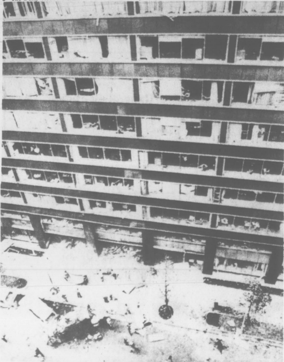
BOMBED —This is the front of the Mitsubishi Heavy Industries Building in the prestigious business district in the heart of downtown Tokyo showing the destructive force of a large explosion which killed at least five people and injured more than 100 today. (AP Wirephoto)
