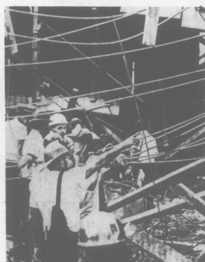
SEARCH FOR VICTIMS —Miami firemen and police search for victims Monday afternoon in the rubble of a motel construction after part of the third floor collapsed. Six workmen were injured, police reported. (AP Wirephoto)
