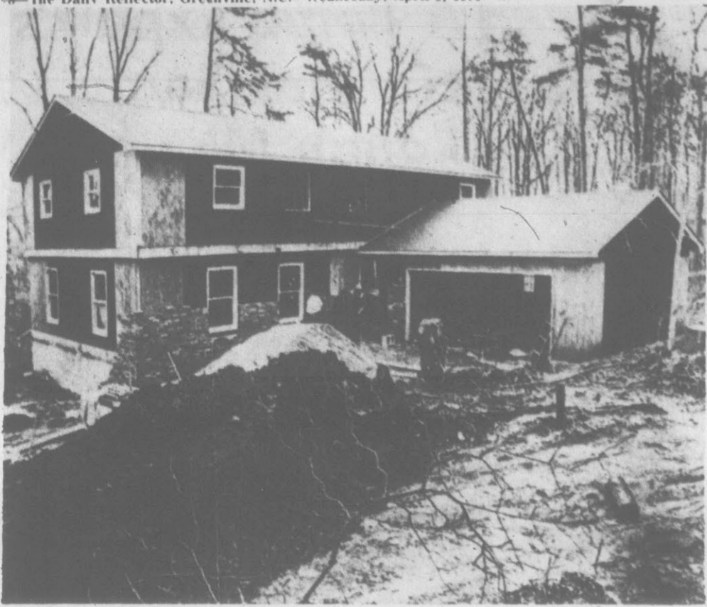
NEW AGNEW HOUSE —This house under construction near Annapolis reportedly has been purchased by Spiro T. Agnew and his wife, Judy. The builder would not confirm which house the
