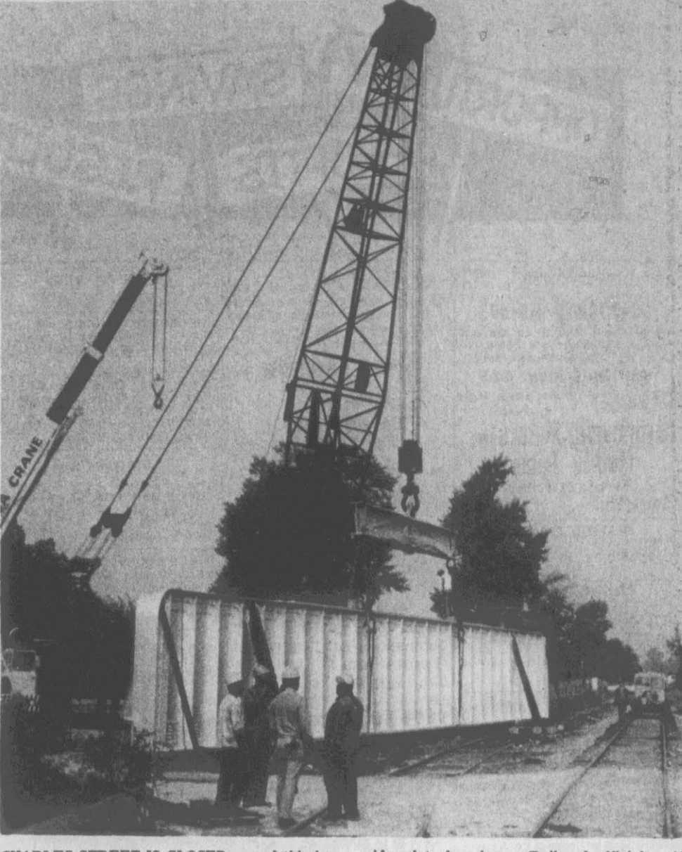
CHARLES STREET IS CLOSED. . . and this is the reason why. Norfolk and Southern Railroad crews are shown readying a 117-ton, 133-foot-long steel beam for loading on flat cars, then to be hauled several hundred feet East to the Charles Street overpass crossing. Charles Street was closed Monday to permit erection of two of the large steel beams which will support the railroad across Charles Street. The street is being widened to four lanes. Railroad officials say they hope to have the beams safely in place by Wednesday night so traffic can be allowed to flow normally again. A 150-ton crane is being used to handle the heavy steel supports. Some 53 steel cross members will connect the two beams and support a deck plate over which the railroad will run. (reflector Staff Photo)
