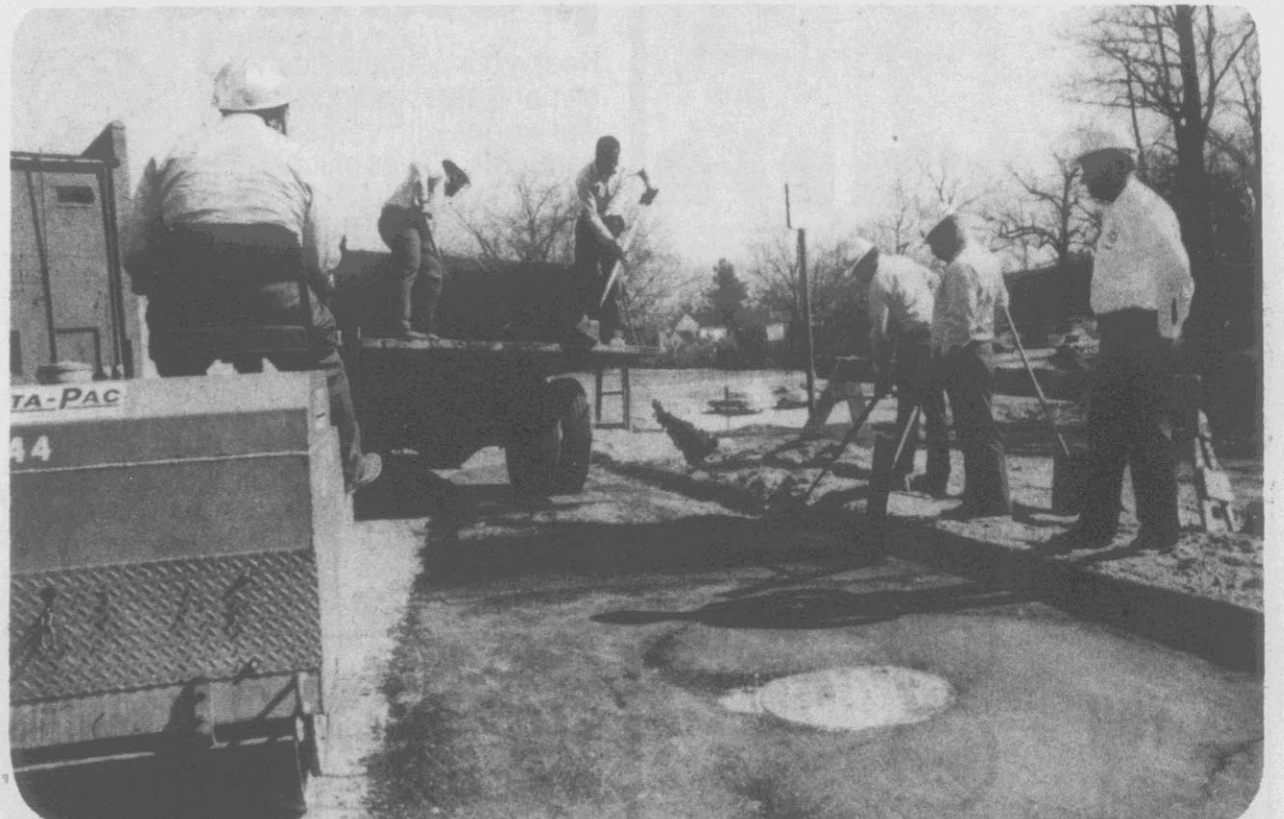
PATCHING A STREET. . . Workers in the Street Department section patch a portion of a worn street in downtown Greenville.
