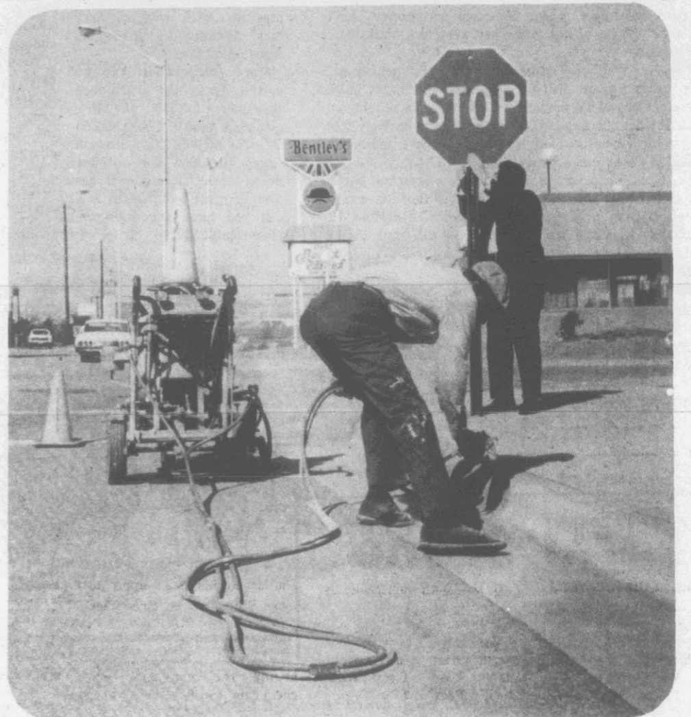
PAINT AND SIGN DEPARTMENT IN ACTION. . . Mark Clemmens paints a curb while Ernest Harris repairs a stop sign.
