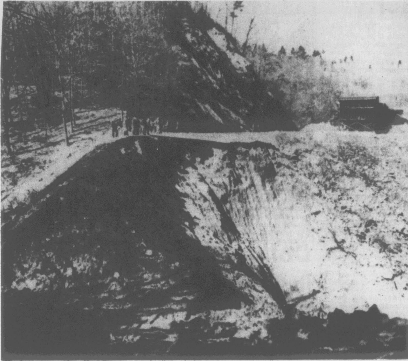
Massive Highway Washout
