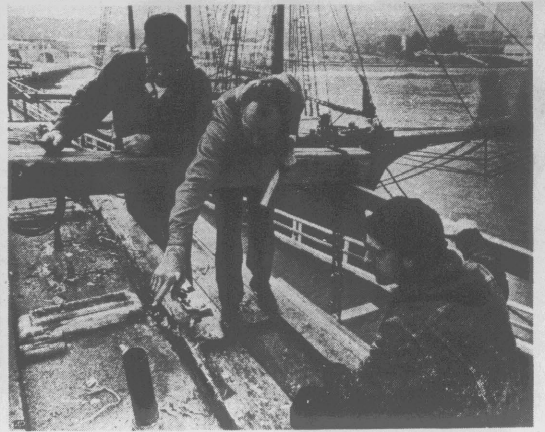
LEARNING HIS TRADE — David Houck, right, said by his union to be the only shipwright apprentice in California, gets a lesson in repairing a cabin on a ship from Ed Doney, left, and Dick Linville. Houck works beside older craftsmen, repairing and restoring the collection of old wooden vessels moored in California's Maritime Historic Park near Fisherman's Wharf in San Francisco.
