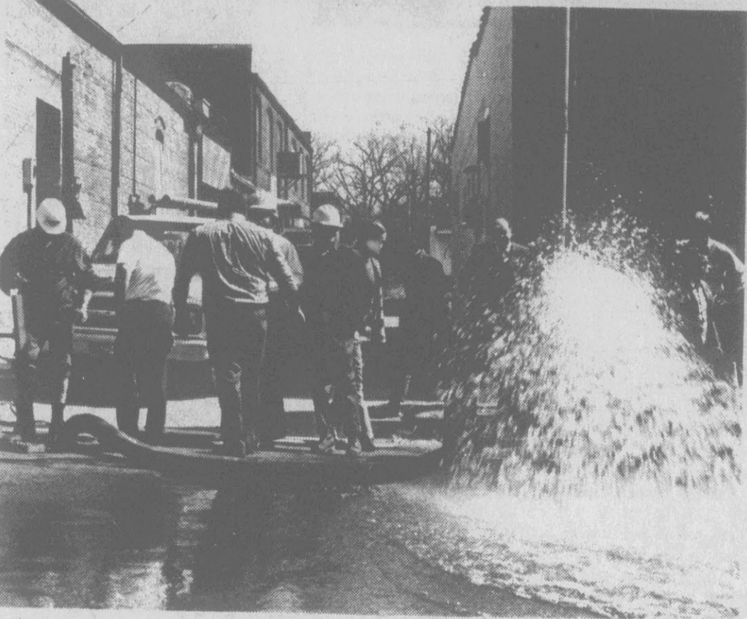
UNDERGROUND WIRES SHORT ... Utilities Commission crews pump water from a manhole housing underground power lines after a short circuit and explosion before Noon Sunday, that caused an interruption of electric service to downtown businesses and churches.
