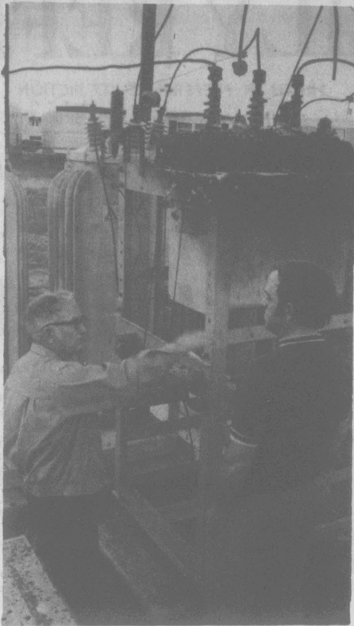
SUBSTATION KNOCKED OUT. Henry Hoell, supervisor of electrical distribution (left) and Malcom Green, assistant Director of utilities, look at a portion of a burned circuit breaker. (Reflector Photo by Tommy Forrest)
